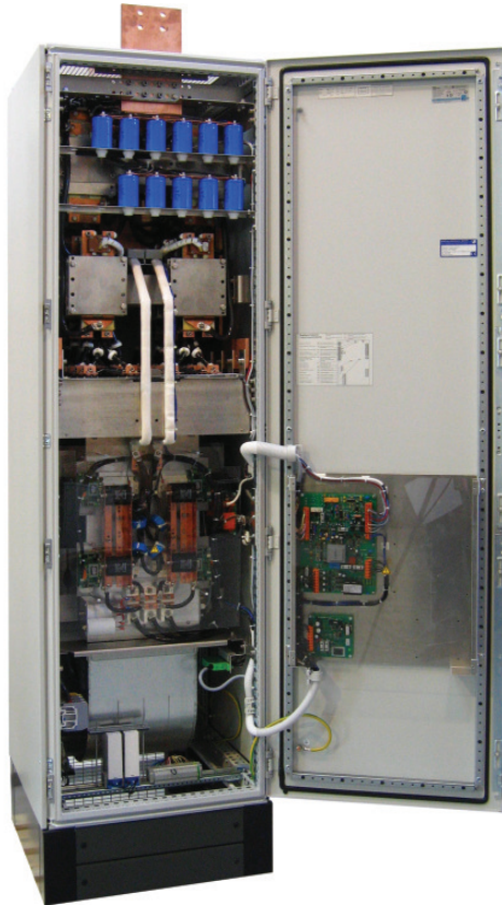
POWER STATION pe5110, front view
